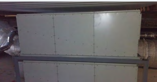
POTOK FED6500 device integrated into the gap of the ventilation channel at the mechanical floor
